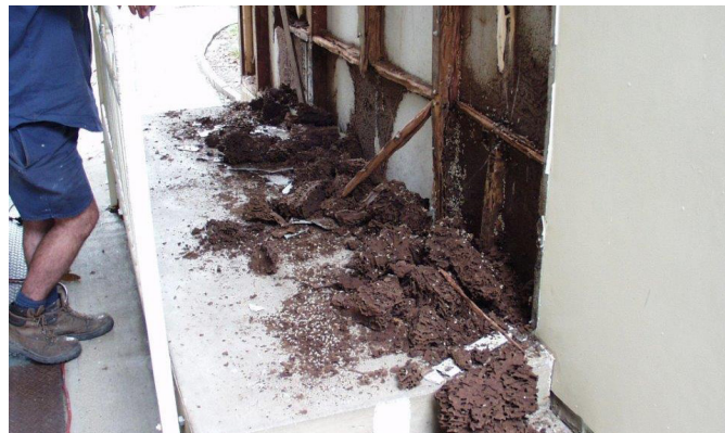
Termite damage can cause a financial burden
